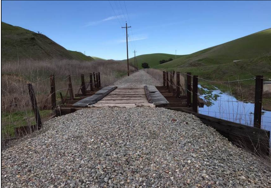
Photograph 17. Culvert 9 wood deck culvert with railroad track side rails, camera facing north, February 6, 2018.
