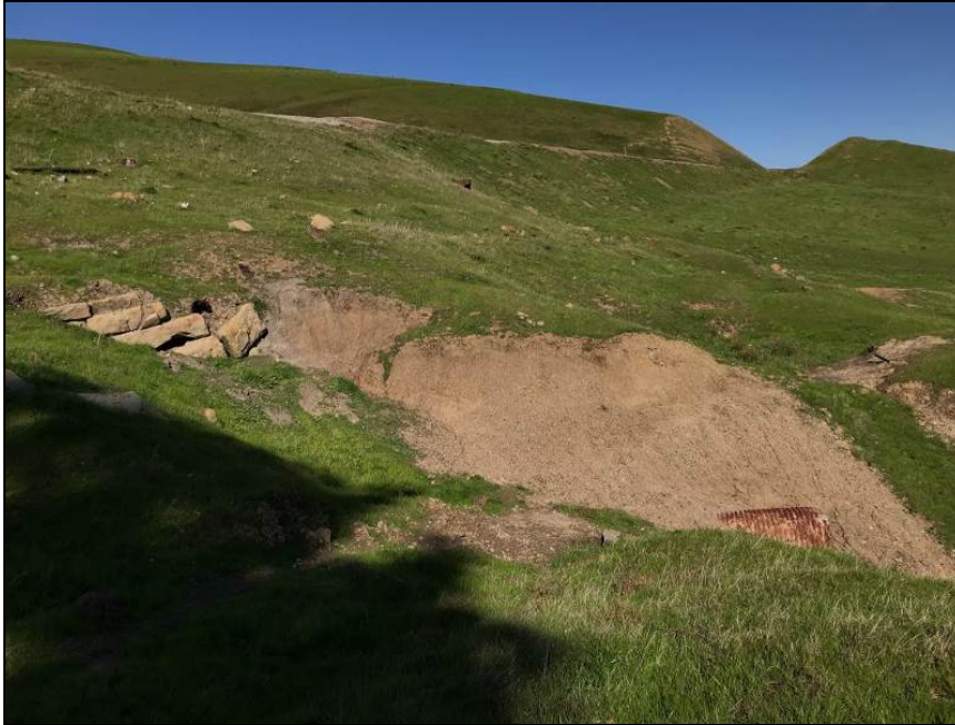
Photograph 15. Culvert 7 sandstone headwall below metal pipe with corrugated metal pipe below, camera facing north, February 6, 2018.
