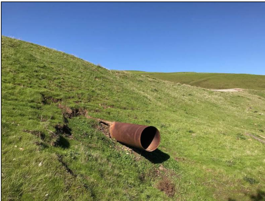
Photograph 14. Culvert 7 metal pipe at south side below railroad grade, camera facing north, February 6, 2018.
