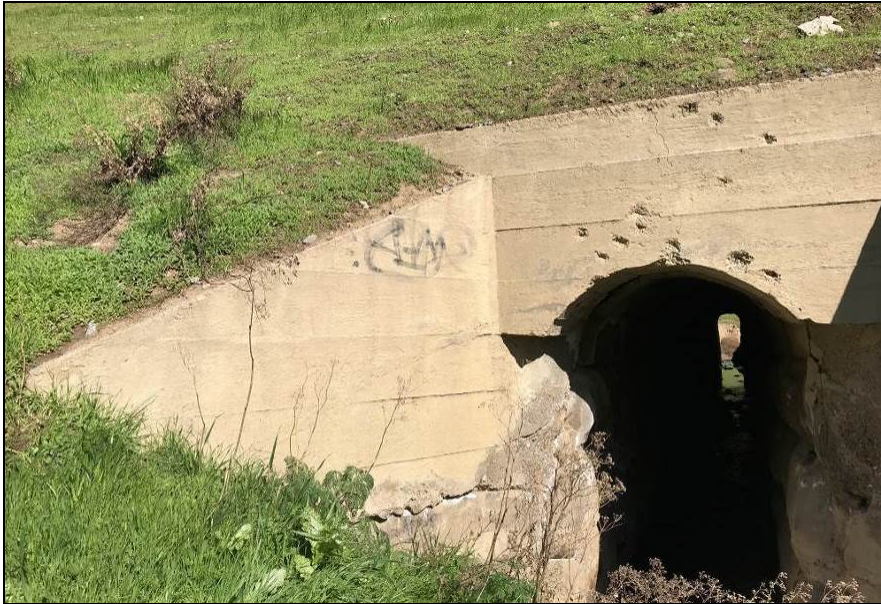
Photograph 13. Culvert 6 southwest side with board-formed concrete skim coat added to headwall and wingwalls, camera facing northeast, February 6, 2018.
