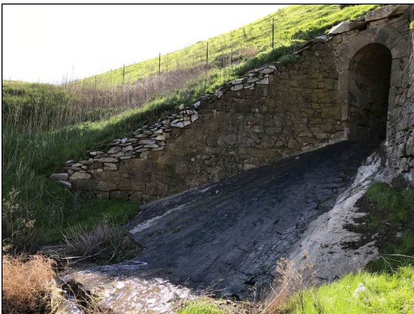
Photograph 10. Culvert 6 southeast sandstone wingwall with granite capstone detail, camera facing southwest, February 6, 2018.
