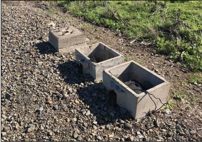
Photograph 29. Signal 2, battery boxes and footing, camera facing northeast, February 6, 2019.
