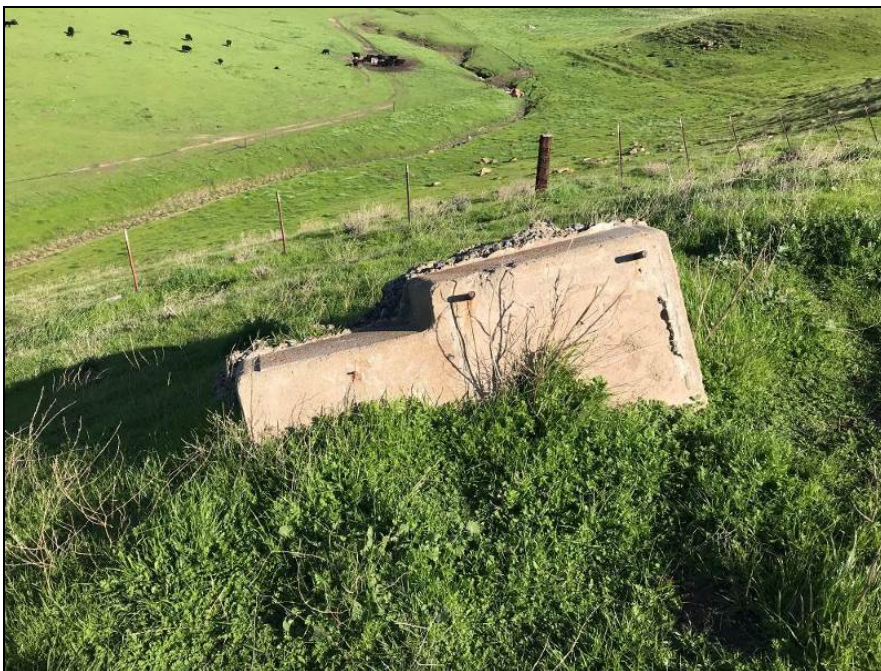
Photograph 28. Signal 1, searchlight signal footing along former railroad alignment, camera facing north, February 6, 2019.
