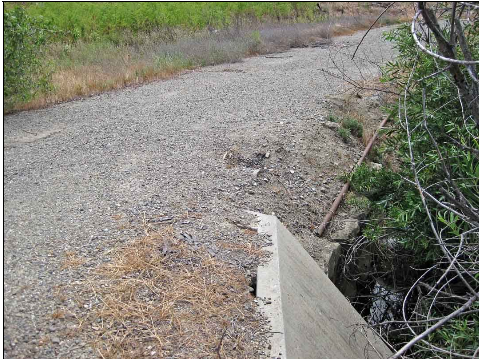
Railroad grade with north side of culvert just beyond modern culvert concrete, facing southwest.
