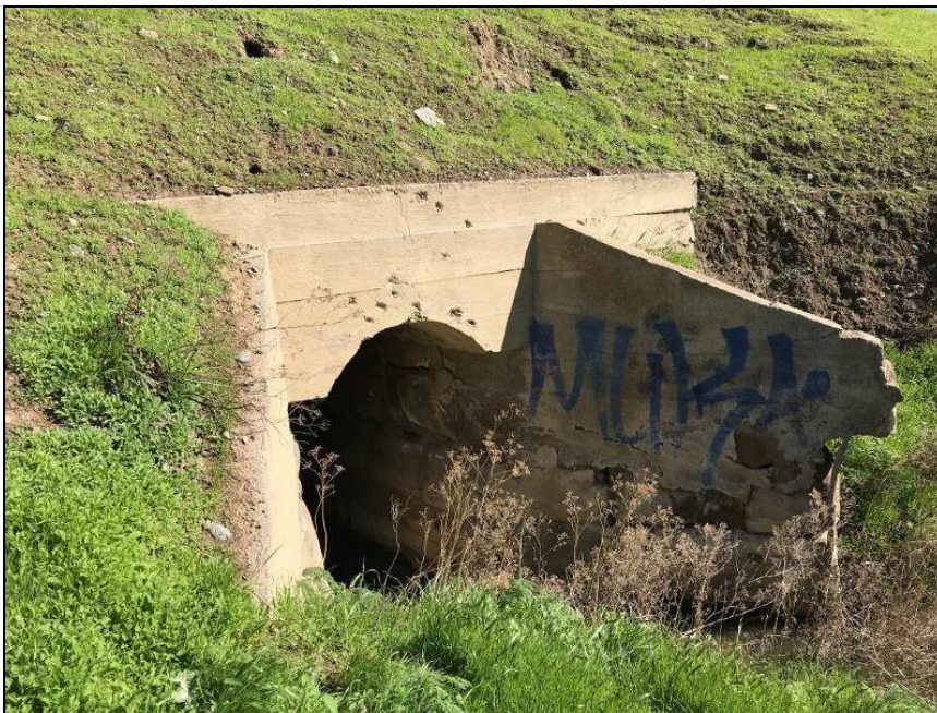
Photograph 12. Culvert 6 southwest side with board-formed concrete skim coat added to headwall and wingwalls, camera facing east, February 6, 2018.
