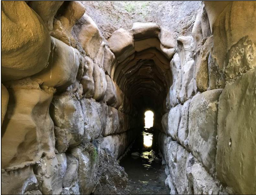
Photograph 11. Culvert 6 view within tunnel of collapsed roof, camera facing southwest, February 6, 2018.
