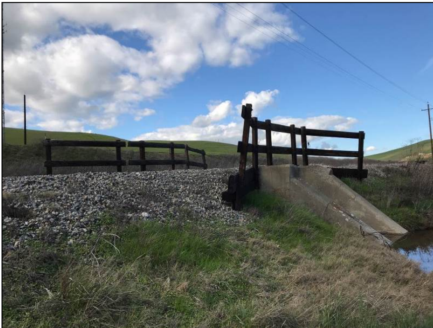
Photograph 16. Culvert 8 concrete box culvert with wood side rails, camera facing northwest, February 6, 2018.
