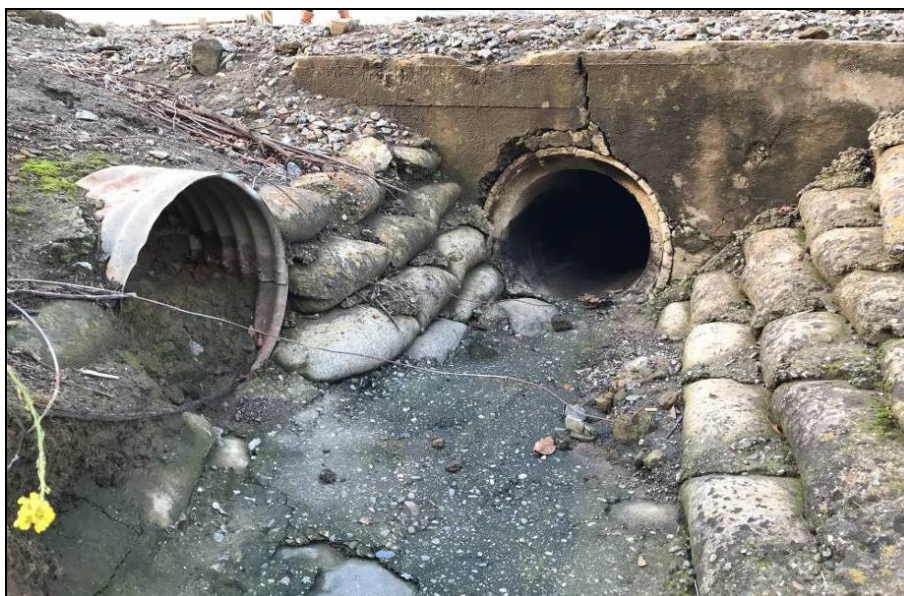
Photograph 20. Culvert 12 concrete headwall with concrete pipe and secondary corrugated metal culvert, concrete bag riprap, camera facing north, February 6, 2018.
